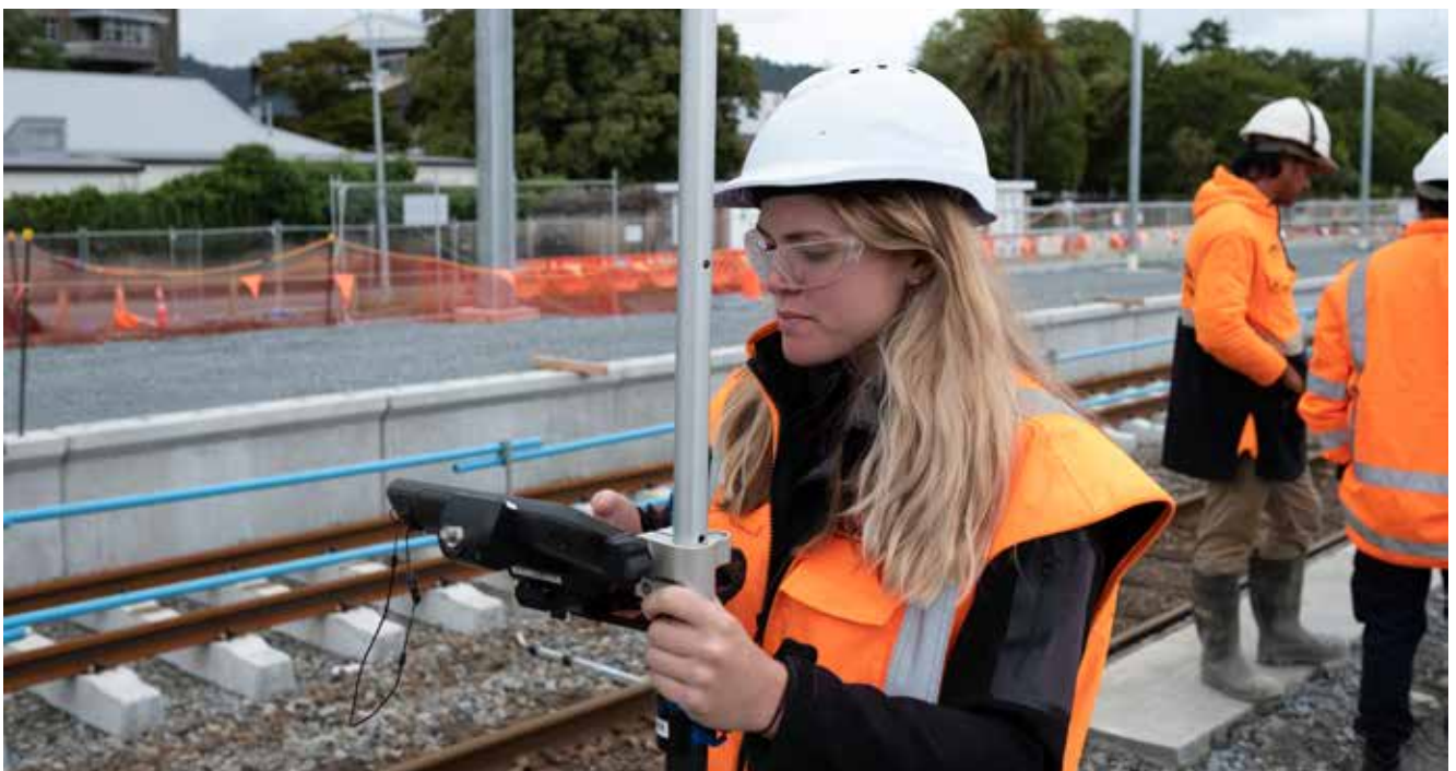
Downer engineer Sarah Doyle is using GPS at Trentham Station to mark out locations for new light poles and underground services. This work is part of the Trentham to Upper Hutt double-tracking project, one of several projects included in a coordinated programme of investment packages to upgrade the Wellington commuter rail network. The works are being funded by Waka Kotahi and the Ministry of Transport.
