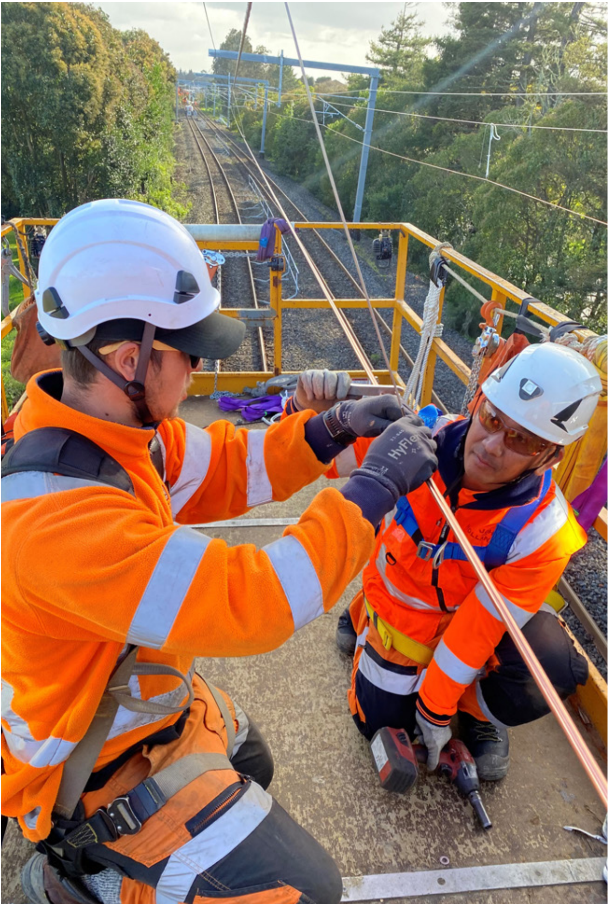
Substantial investment on the network continues, including on the overhead used to power the commuter units to make sure it is resilient and delivers for passengers.
