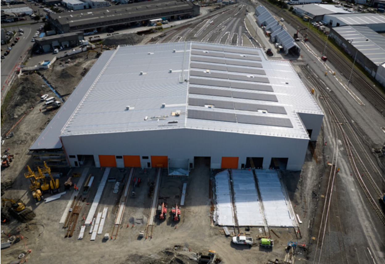
Installing solar panels at the new mechanical hub at Waltham, Christchurch, is part of KiwiRail’s commitment to decarbonisation.
